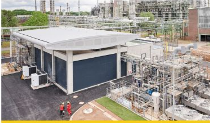
Our 10 MW proton exchange membrane (PEM) electrolyser in Germany.
