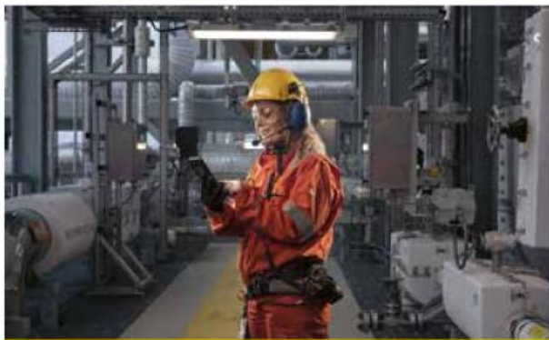
The Nyhamna gas plant processes gas from the Ormen Lange field, 120 kilometres off the Norwegian coast.
