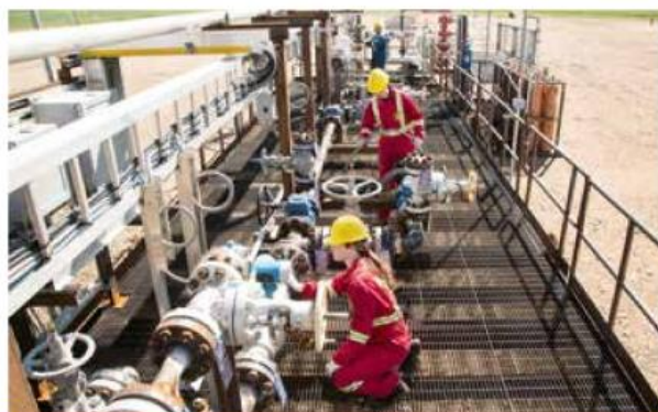
The Quest CCS facility in Alberta, Canada.
